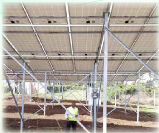
The new solar powered Ex-pages borehole project in Mweiga ward, Kieni West sub county.
