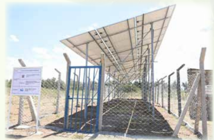
Gitero Solar Powered borehole in Narumoru / Kiamathaga ward, Kieni East sub county.
