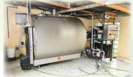
The recently installed milk cooler at Mathaita Farmers Cooperative Society in Narumoru / Kiamathaga ward, Kieni East sub county. This will help improve quality and quantity of milk in the area.
