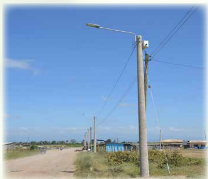
Newly installed street lights at Kwa J trading centre in Thegu River ward, Kieni East sub-county.
