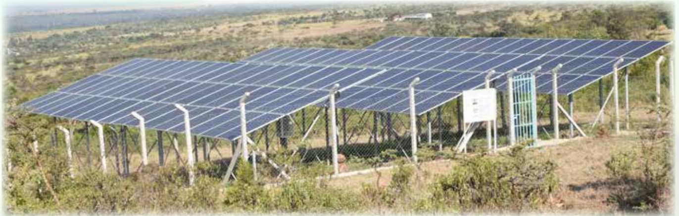
Solar powered Kienjoro borehole project in Mugunda Ward, Kieni West sub county.
