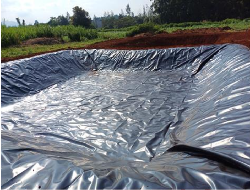
Lined water pan for water harvesting at Wambugu ATC
