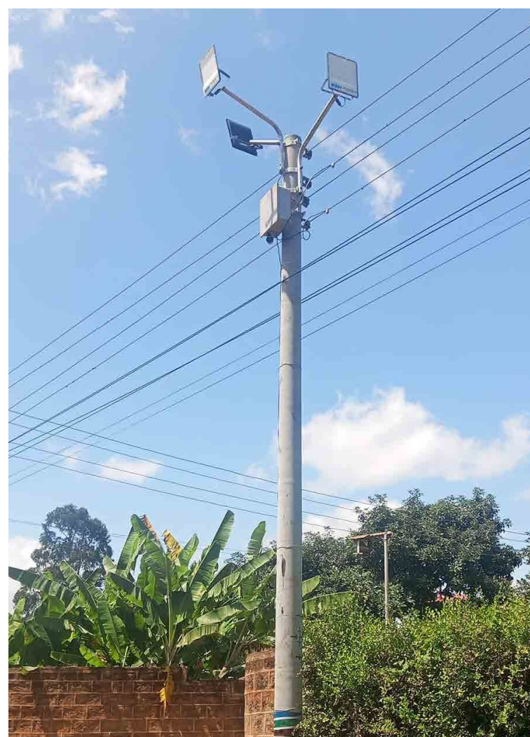
Installed stand alone street light along Classic - Muthaiga - Ngangarithi road.
