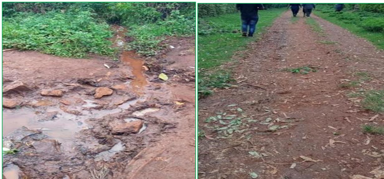
Plate 17: Storm Water Drainage
