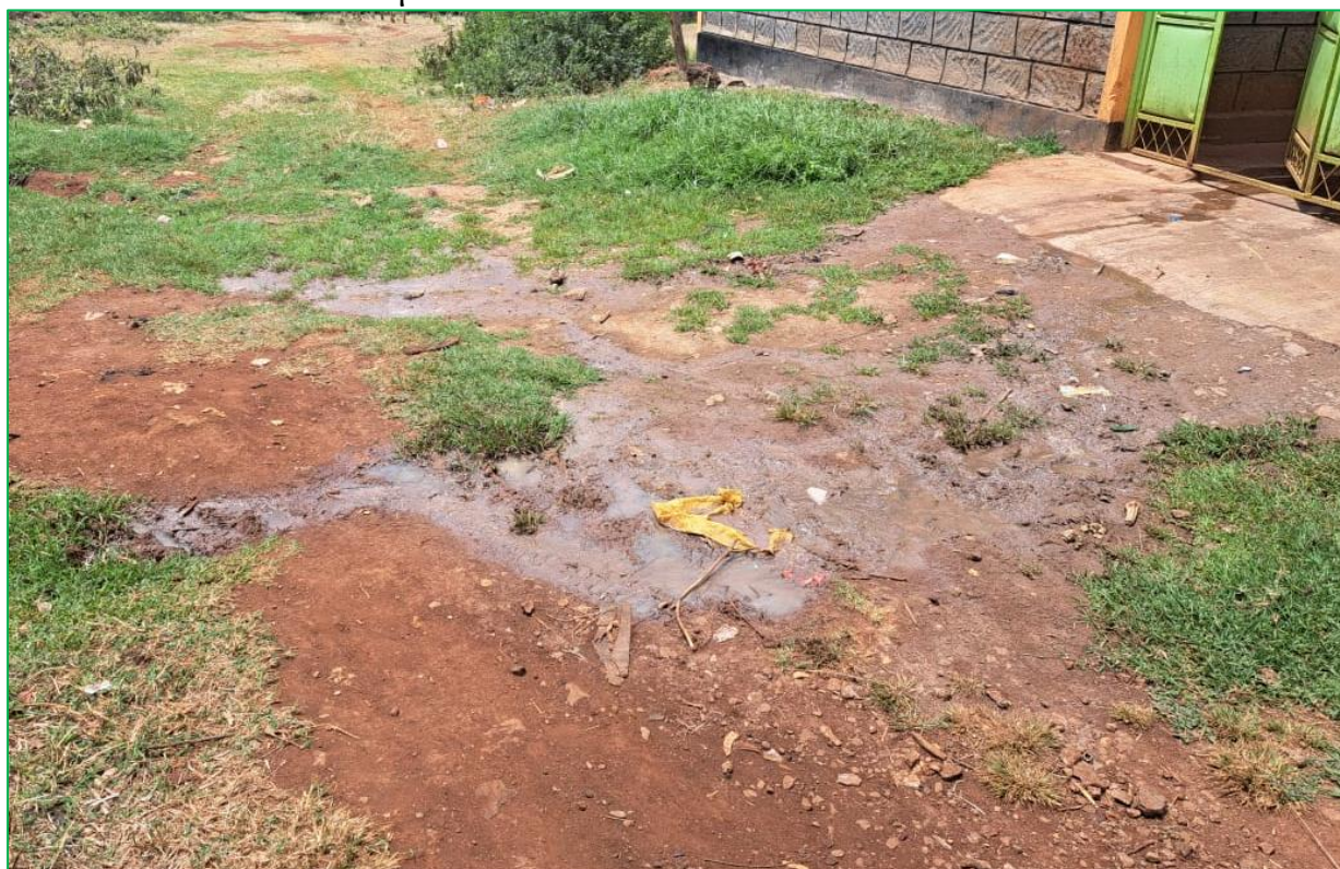
Plate 12: Waste Water Disposal
