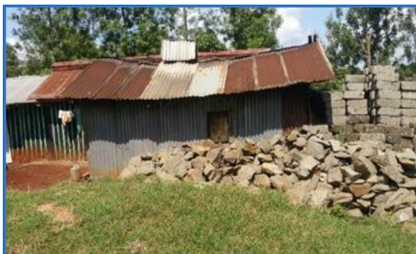
Dilapidated temporary house
