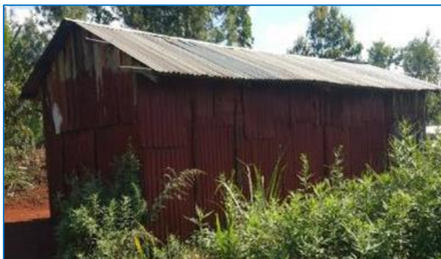
Dilapidated temporary house
