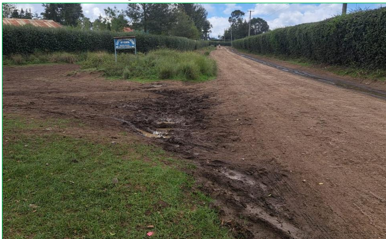
Plate 11: Storm Water Drainage
